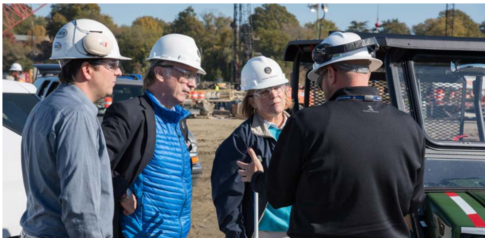
On Friday, Nov. 18, Ben Duman (O41), left, and Director of Facilities Lucas Hicks , right, gave Greg Willard, center left, and Susan Ford Bales , center right, a tour of the construction site for the new Joint Manufacturing Assembly Facility. Photo by Ashley Major
