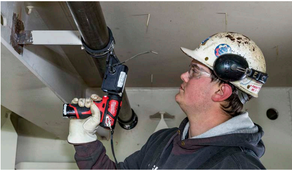
Christopher Eckstein uses the new pipe-banding system on John F. Kennedy (CVN 79). Photo by John Whalen
