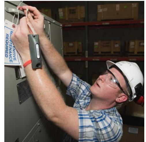
Kyle Davis (O52) installs a tag that will track an asset as it is moved around the shipyard. Photo by Ashley Cowan
